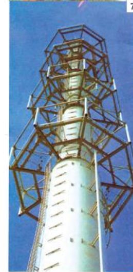
7 Maintenance platforms for the Talk Tower in Lafarge (Egyptian Cement)
